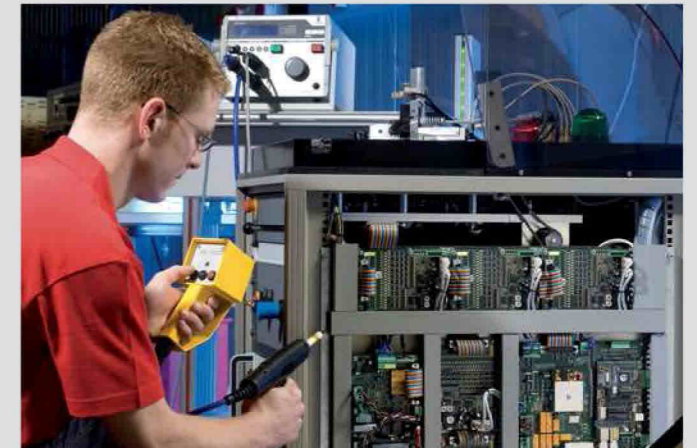
EN60204 test at a service cabinet
